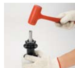
10. Push the other bearing out by rubber hammer
